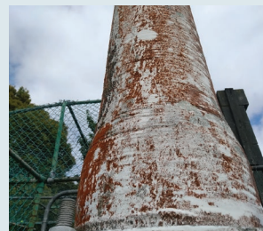
Deteriorated light poles
